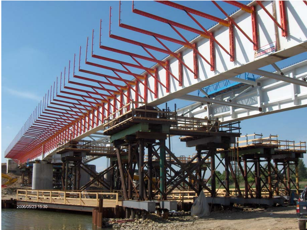
Mounting of the form panels onto the main girders web, in front view the yokes used also for concreting in May 2006
