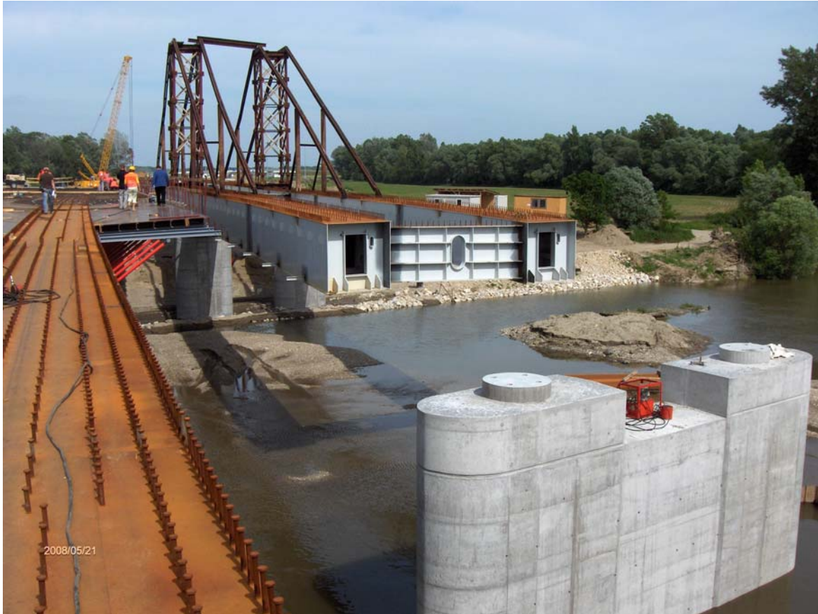
Longitudinal launching in 2008, form paneling of the rc deck slab of the other bridge
