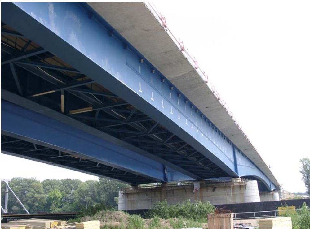
River bridges view from the bottom, after removal of the form panels
